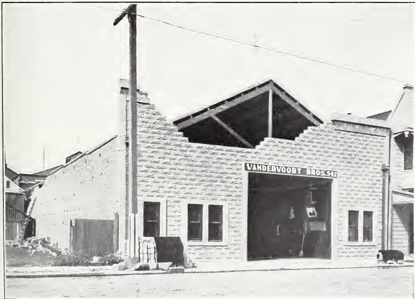
B. WALL THROWN DOWN BY EARTHQUAKE VIBRATIONS OF ROOF TRUSSES WHICH WERE NOT TIED TO WALL, VANDERVOORT BROTHERS' LIVERY, PALO ALTO.
